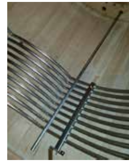
MLP sensors inside the tank.
